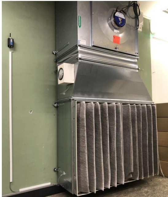
Figure 9: Filter system equipped with LoRa monitoring sensor module (PRiOT AG)
