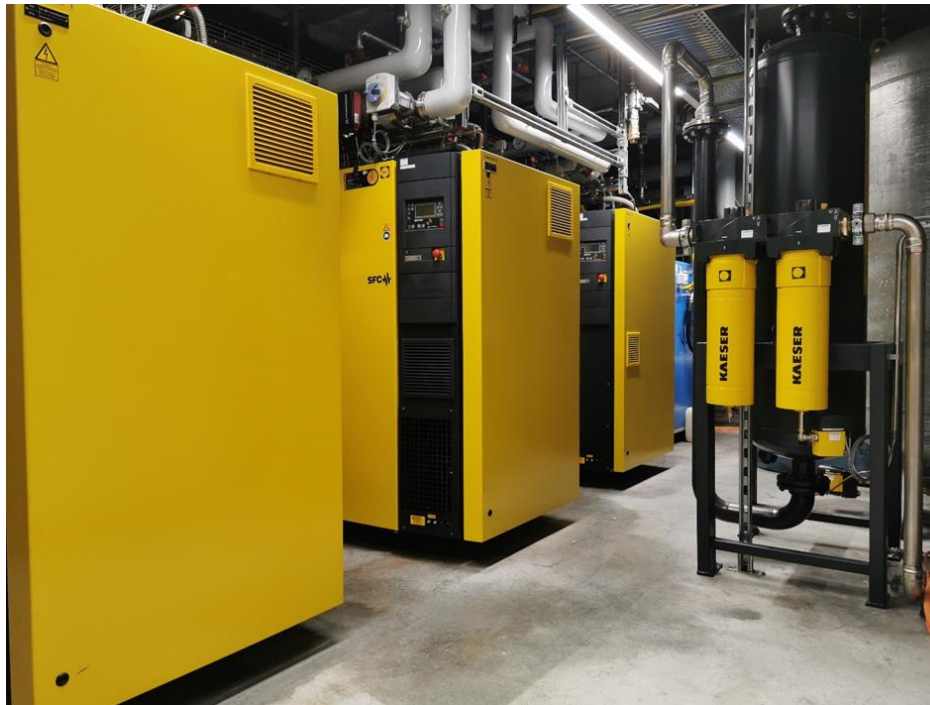
Figure 21: Air compressor system (Picture: Pascal Kienast)
