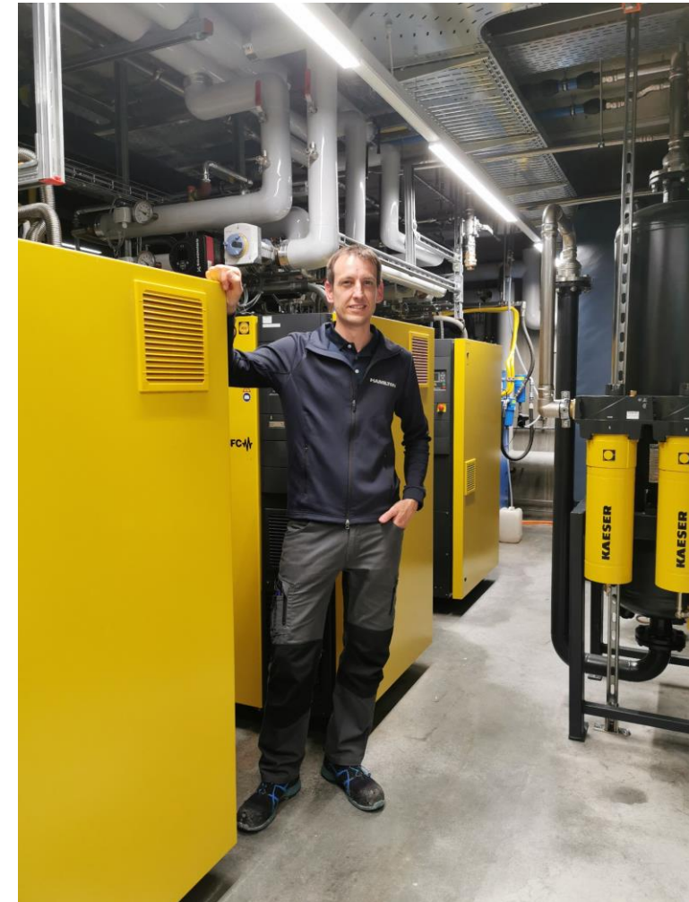
The new compressed air system with Achim Sax, Director Facilities Hamilton Services AG (photograph: Pascal Kienast)
